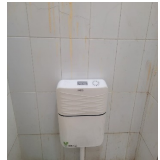
Dual flush system installed
