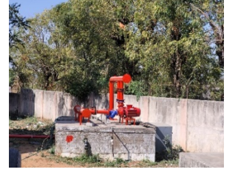
Fire water tank
