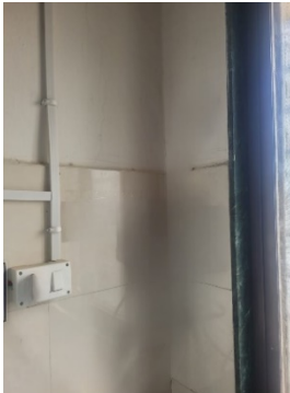
No water Alarm System
