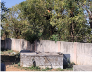
No fire water tank
